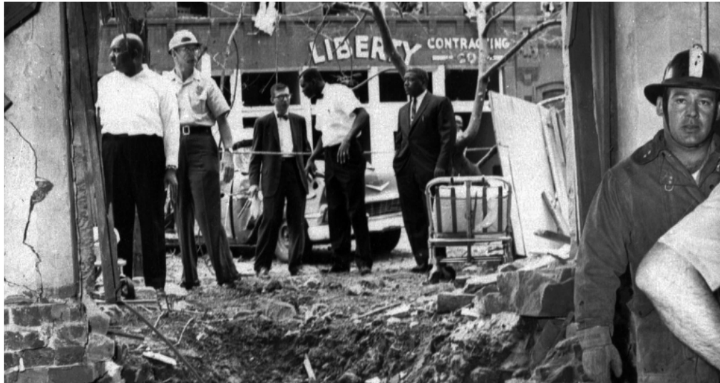
The crater and other damage caused by the bombing of the Sixteenth Street Baptist Church, which killed four African-American girls. AP Photo.
